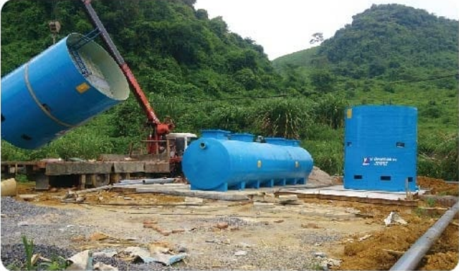
WWTP – Thuy Phuong Pig Farm – Hoa Binh
