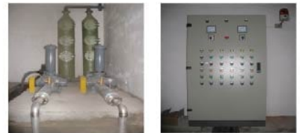
Air blower and Control Panel
