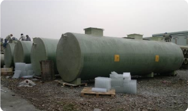
WWTP – Thuy Khue Flower Village – Ha Noi
